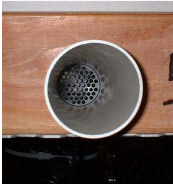
Figure 6. End view of boot leak showing the PVC plug used for the register closing tests.
