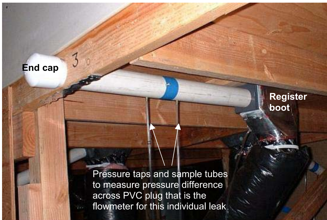
Figure 7. Boot leak showing end cap and attachment to boot.
