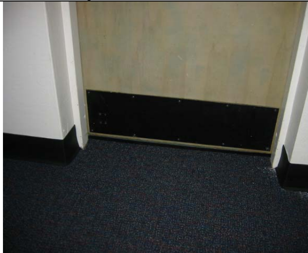
Doorway to enclosed stairwell is not weatherstripped.
