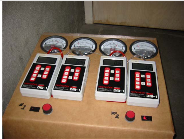
Gauges measure the pressure on each floor as well as the flow from each fan.
