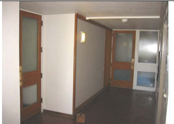
Lack of weatherstripping on double doors at the end of the hallway would allow smoke from the lobby to enter the apartment areas.
