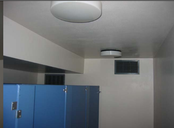
Active and passive returns in toilet area
