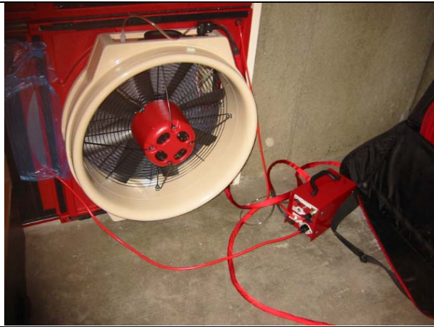
2 HP fan on Variable Frequency Drive mounted from stairwell side ready to depressurize the floor.
