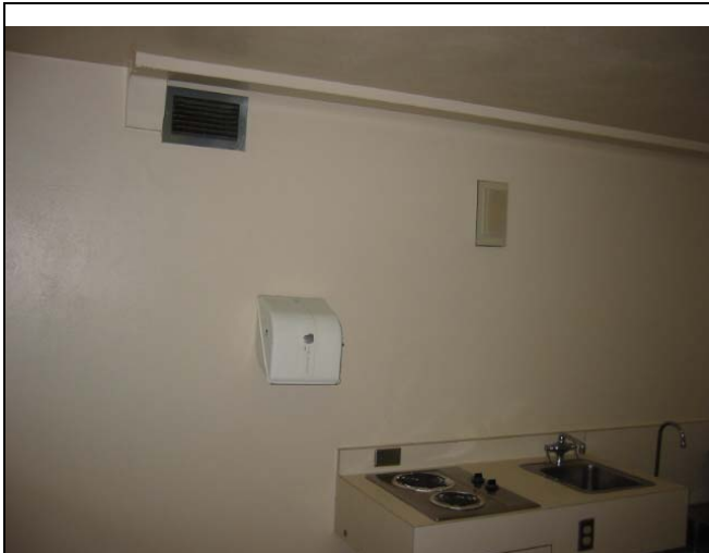
Small exhaust grille for kitchenette
