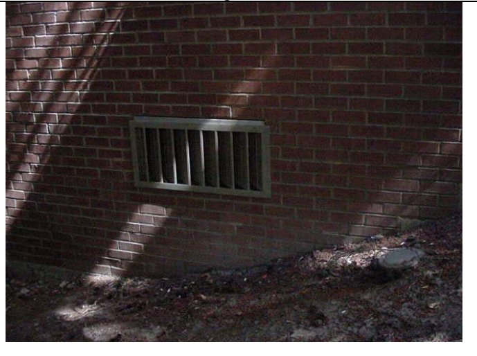
Exhaust vent at ground level.
