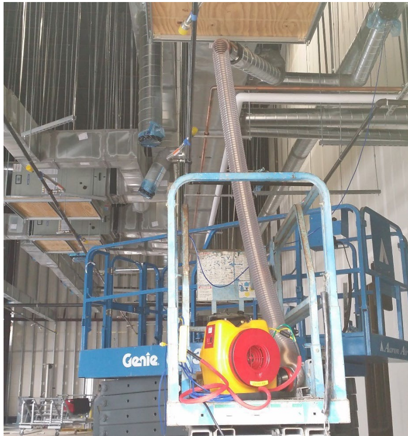
Figure 10 Model 500 Blower set up to test ducts prior to installation of the Flow Plug that is needed to measure flow.
