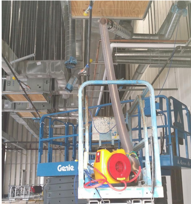
Figure 10 Model 400 Blower set up to test ducts prior to installation of the Flow Plug that is needed to measure flow.
